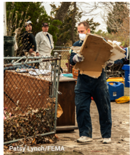
Volunteers help clean up a Union Beach neighborhood after Hurricane Sandy.
