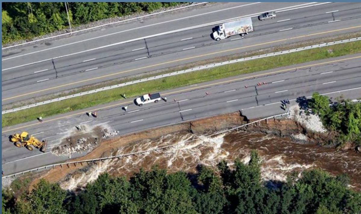
Route 287 in Morris County – Northbound shoulder washed away by floodwaters from Hurricane Irene
